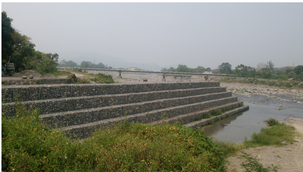
Figure 11. Breakwaters built near the bridge to protect it from the river current.
